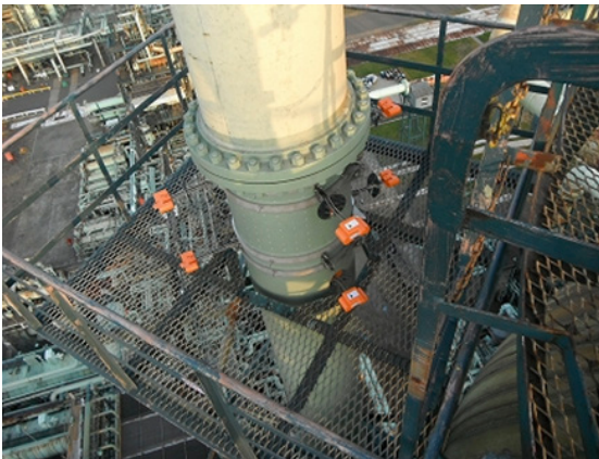
Figure 7 Idemitsu site installation picture.
