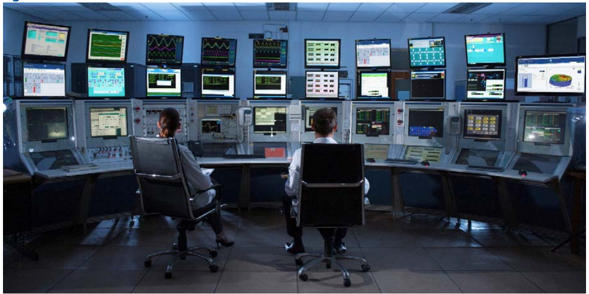
Figure 1-2. View of Control Room
