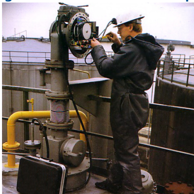
Figure 6. Reduce Maintenance Spending and Improve Safety
