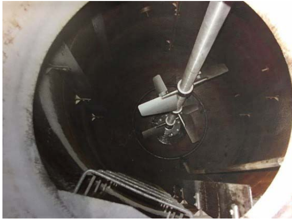
Figure 4. The Internal of the Tested Vessel
