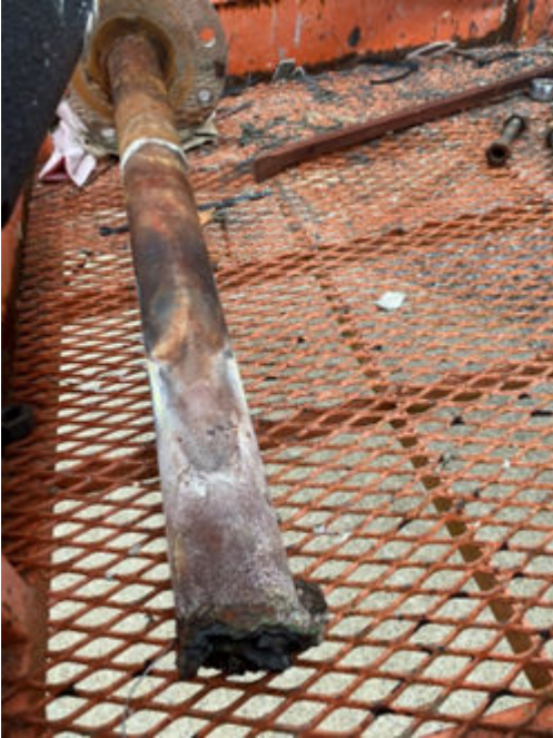
Figure 7: Bypass Nozzle Corroded Away Preventing Sample Flow
