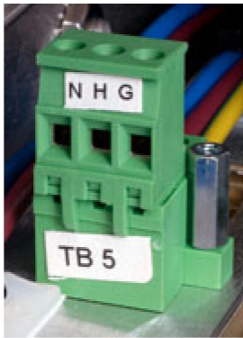
Figure 3-9: AC/DC termination block
