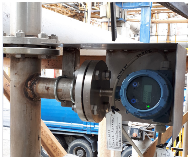
Fork Density Meter, 2" pocket recessed installation at the chemical plant.
