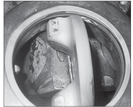
Figure 1 - Valve properly clamped in place.
