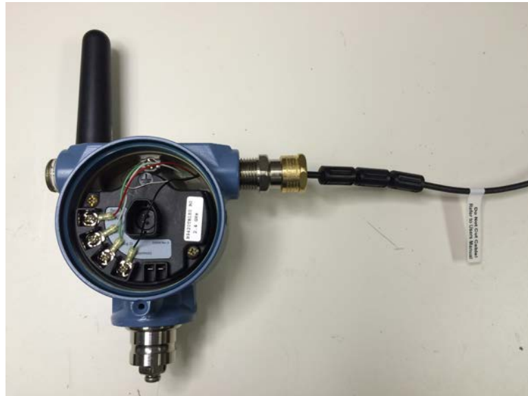
Figure 6-7: Ferrites installed on a standard cable
