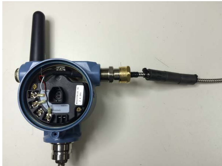
Figure 6-8: Ferrites installed on an armor-jacketed cable
