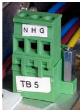
Figure 5-8: AC/DC termination block
