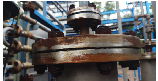
Unmonitored corrosion can cause expensive downtime.
