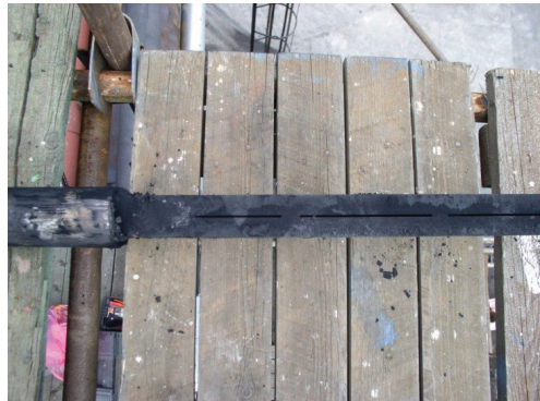
Figure 10.44: Close up of the solids buildup on the base of the Stack Annubar sensor exterior. Required maintenance is needed to clean the sensor periodically.
