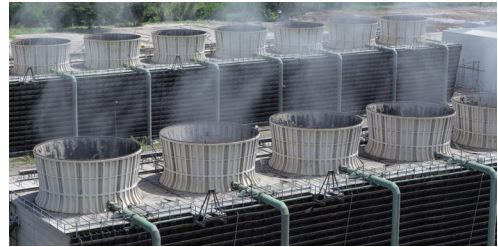
Figure 5.2: An industrial cooling tower, which uses evaporation of water to remove large amounts of heat from an industrial process.
