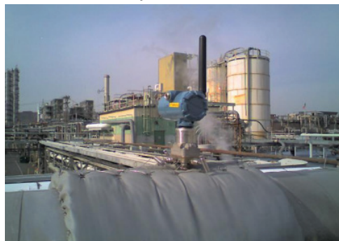
Figure 10.15: Direct mounted Rosemount 3051SFC wireless flow meter on an exterior steam application where the steam temperature is 365 °F (186 °C).
