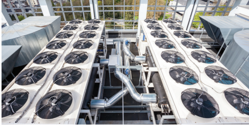
Figure 4.9: An air-cooled chiller for an air conditioning system.
