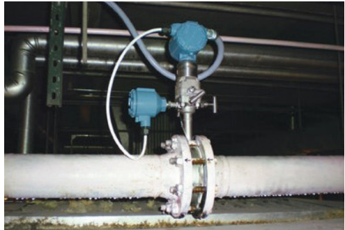
Figure 4.4: A Rosemount Compact Annubar™ Flow Meter installed in a natural gas line at a pulp and paper mill.
