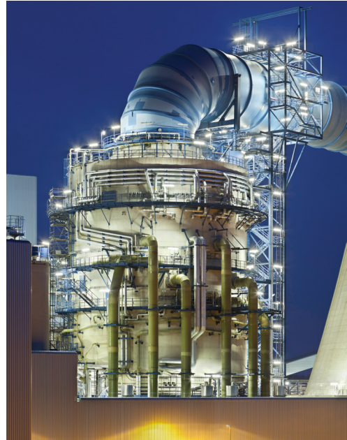
Figure 4.10: A utility scrubber for emissions reduction.
