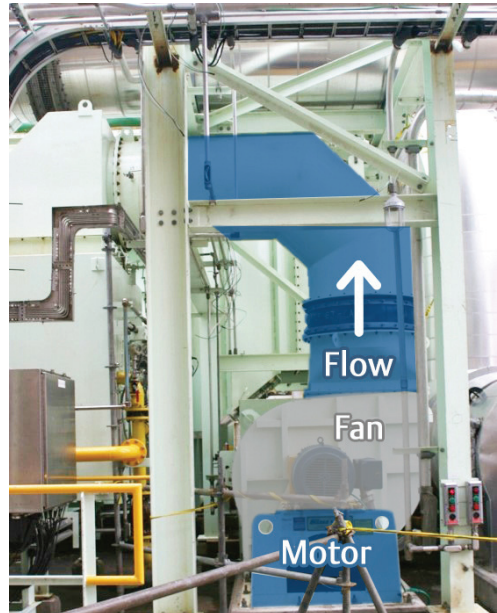
Figure 4.7: A boiler forced-draft fan for combustion air flow.
