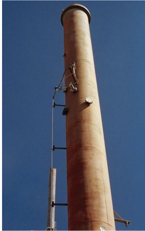
Figure 10.43: Stack primary element removed from a stack to be cleaned. Even with significant buildup of solids on the Annubar Averaging Pitot Tube, the sensing ports remained clear.
