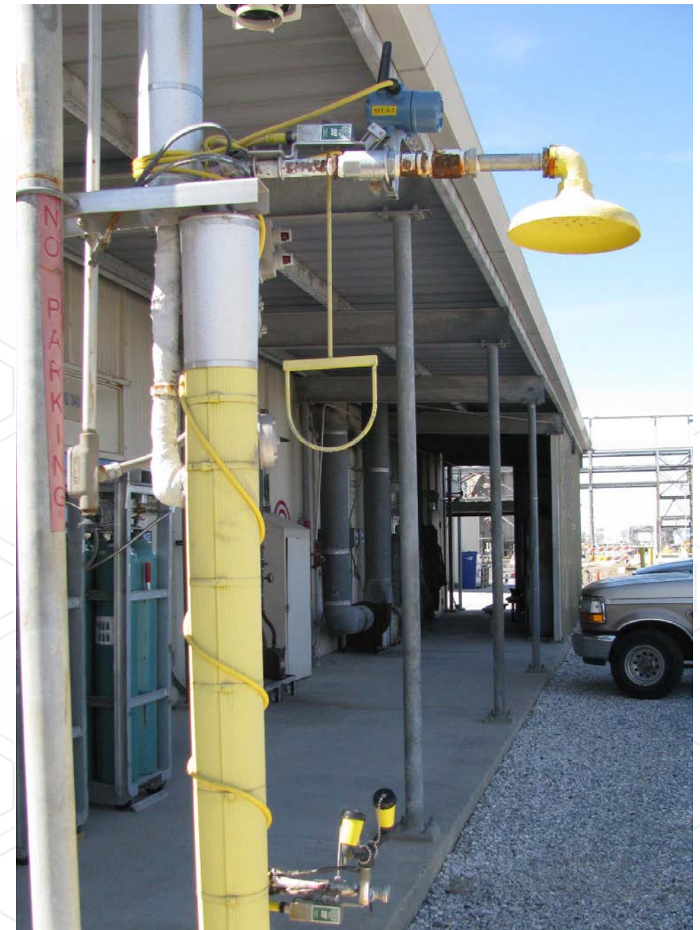
Figure 8: Adding a Rosemount 702 Wireless Discrete Transmitter can tell the control room which safety shower or eyewash station has been activated.
