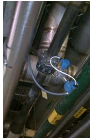
Rosemount Compact Annubar Flow Meter installed between two raised-face flanges
