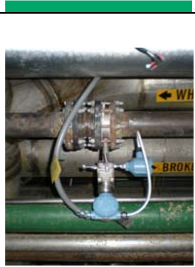
No new piping modifications or welding was required in this quick installation
