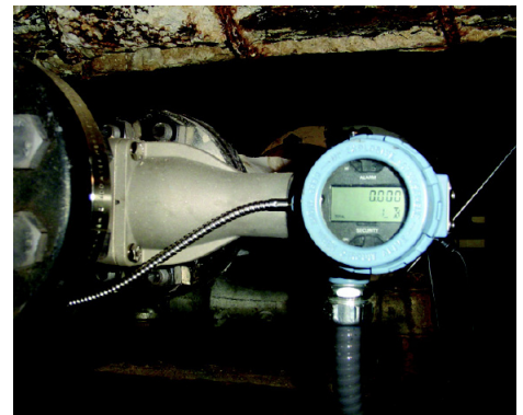
We Energies' Rosemount 8800 MultiVariable steam installation
