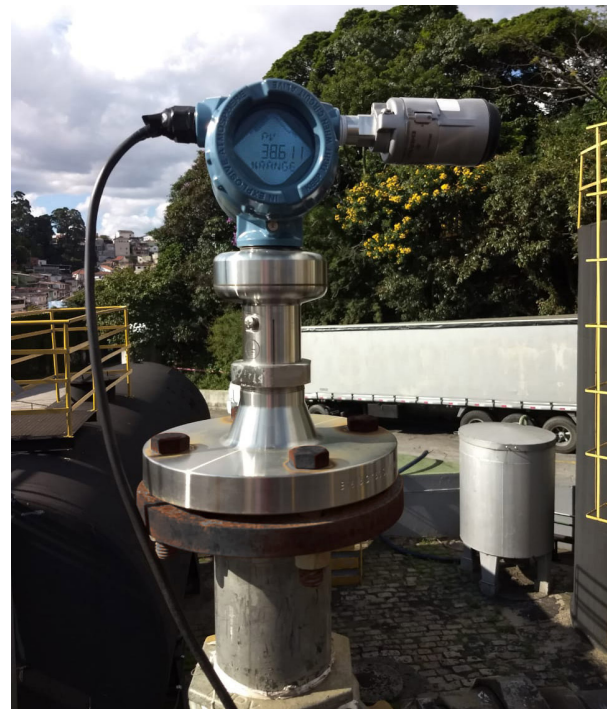
Rosemount 5408 with Emerson THUM Adapter is installed on the asphalt tank
