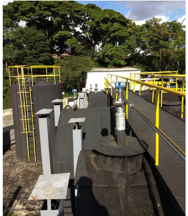
Rosemount 5408 is installed on each tank
