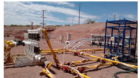
Image 2. The Roxar 2600 Multiphase Flow Meter installed on a well pad in Vaca Muerta
