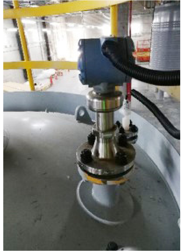
Rosemount 5408 installed on chemical storage tank
