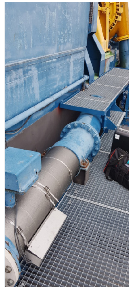
Measuring point on the dredging vessel. Typically, the concentration measurement is not done on the vessel due to the restricted space and the high costs of radiometric instrumentation.
