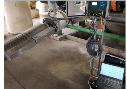
Complete working measuring point in Sibelco's production hall. The clamp-on ultrasonic transducers of the PIOX® S measuring system are mounted on the pipe next to the existing flow and radiometric density measurements.
