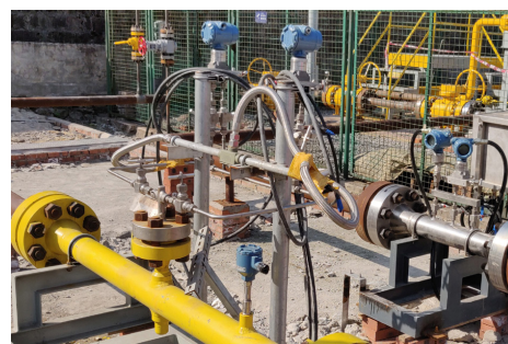
Top: Rosemount 3051S Multivariable transmitter fitted with impulse lines and Rosemount Annubar mounted on the yellow pipe carrying LNG in the underground facility
