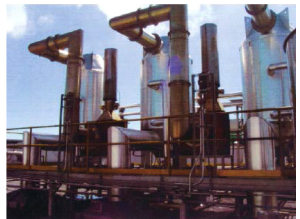
Steam generator capture gases that would be exhausted and use that heat for boiler systems.
