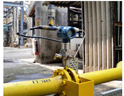
Wireless gas flow measurement with Rosemount Conditioning Orifice Flow Meter and THUM was easily integrated into the plant DCS.
