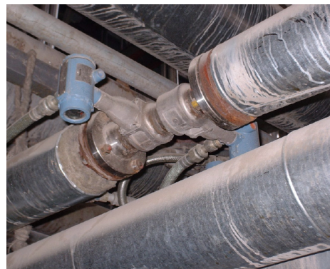
A Rosemount 8800 Dual Vortex installed in a steam line.
