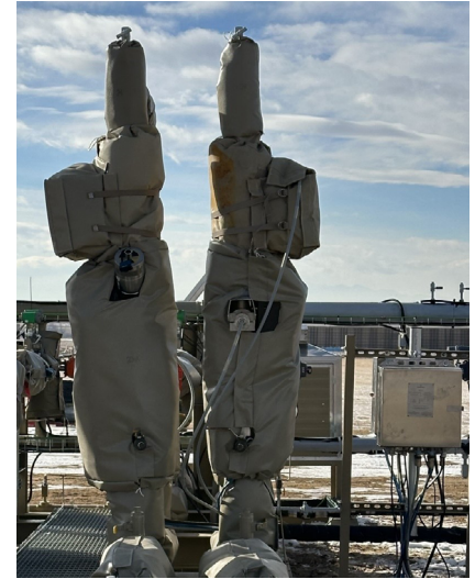
Image 2. Insulated Roxar 2600 MPFMs installed at a well pad in the DJ basin
