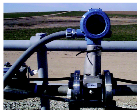
Installed Rosemount 8800 Vortex Flow Meter
