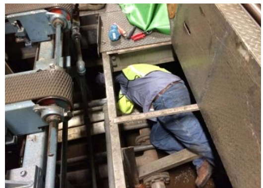
Manual steam trap monitoring can be difficult, as in the case of the “pits” at the tire plant, and always includes working near live steam.
