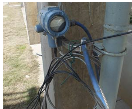
Installed Rosemount 8800 Vortex Flow Meter
