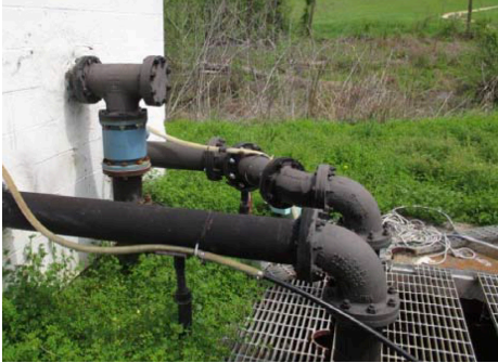
Flow meter installed in the discharge line leaving the station.
