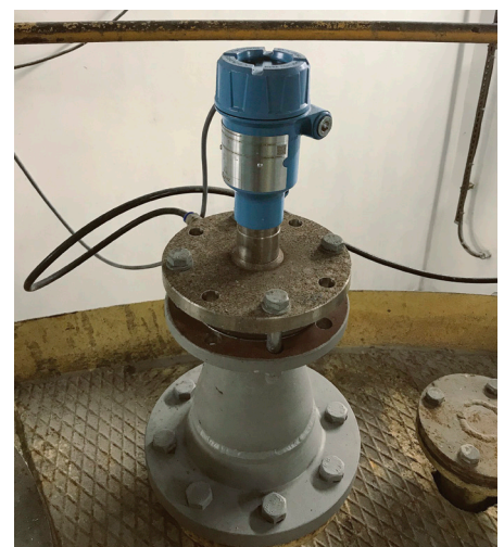
Image 1. Rosemount™ 3408 Non-Contacting Radar Level Transmitter installed on the fine ash silo
