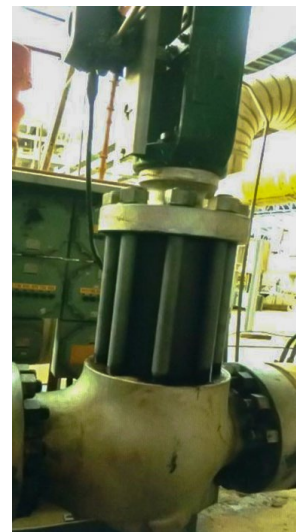
Figure 2. Retrofitted Fisher DST utilized a 4-stage trim
