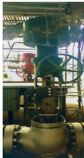
Figure 1. Original valve utilized an HP Cavitrol III 3-stage trim facing clogging issues
