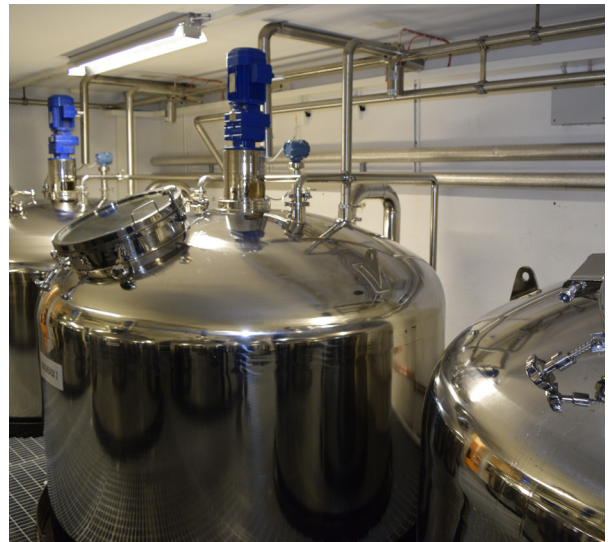
Rosemount 5408 installed on the fermentation tank
