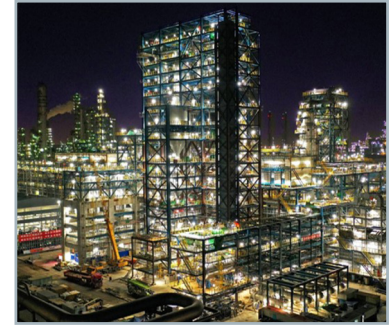
The new Hydrocracking Unit by night
