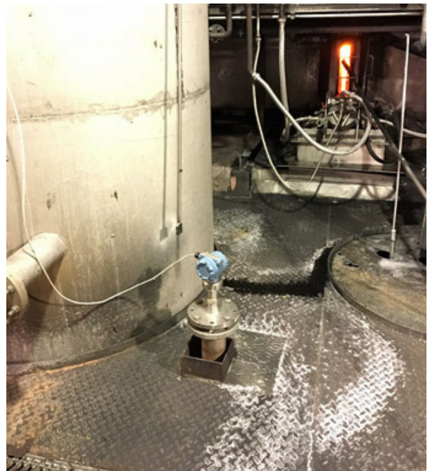
Rosemount 5408 with a process seal installed on the smelt tank.
