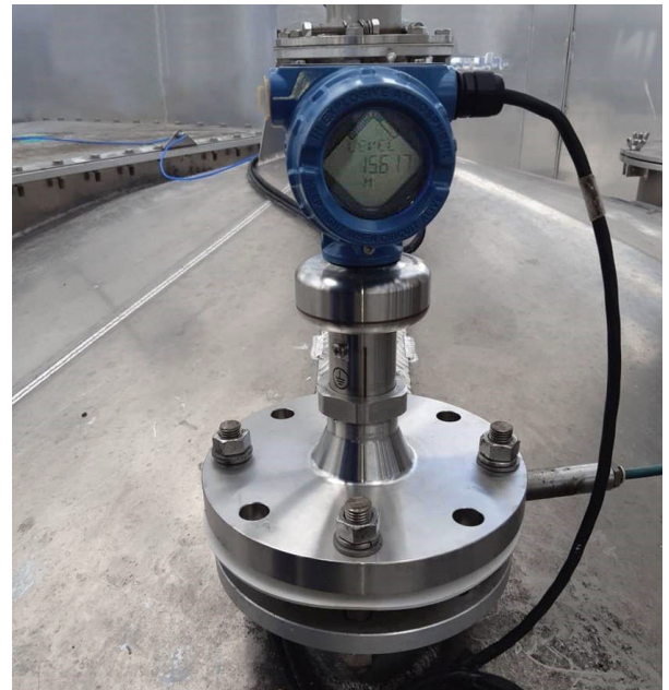
Rosemount 5408 installed on the flour silo
