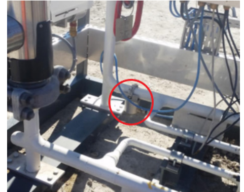
Image 2. The Roxar Acoustic Sand Monitor installed on the skid arrangement for the Roxar 2600 MPFM
