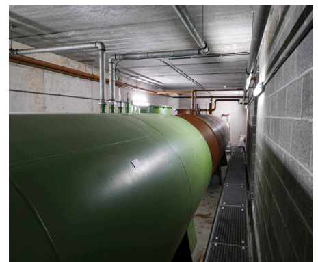
Image 1. Storage bullet tanks containing fuel for planes
