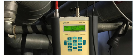
An indispensable tool for the energy experts at Optima for years: the portable FLUXUS® G601 CA Energy.
