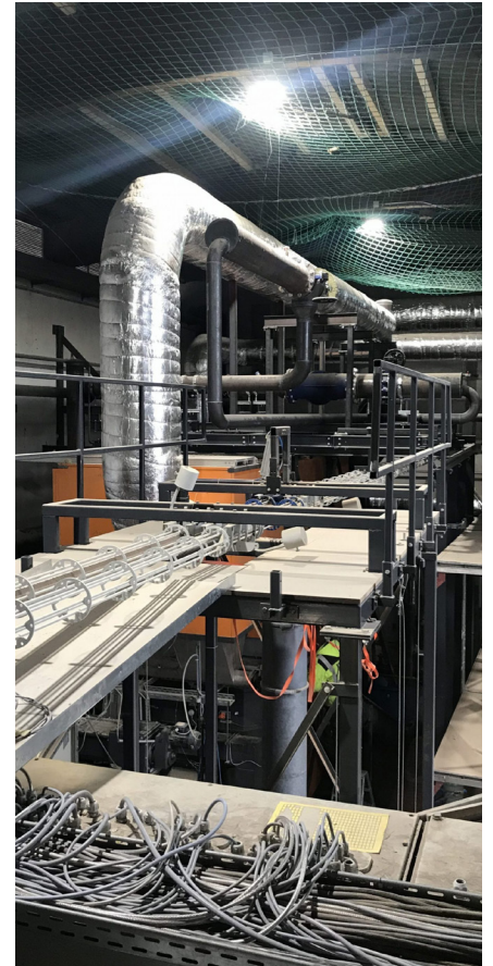
The heating center of the furniture factory during the modernization work.
