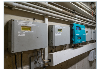
Right from the start, i.e. since 2012, the Elmos combined heat and power plant has relied on non-intrusive flow and heat flow measurement with FLUXUS®.
