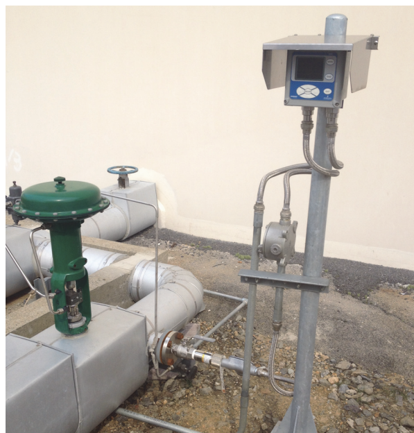
Hydrocarbon leak detection handled by reliable Rosemount 1066 Transmitter and 402 Conductivity Sensor
