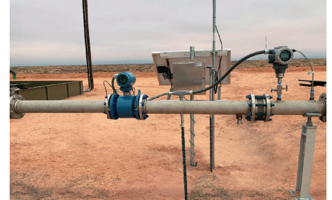
Installed Rosemount 8705 Magnetic Flow Meter (left) paired with the Emerson FB1200 Multi-Run Explosion-Proof Flow Computer for Gas and Liquids (right).
