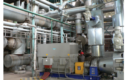
An installed Rosemount DN300/12-in. Magnetic Flow meter to monitor the water flow and pump performance.
