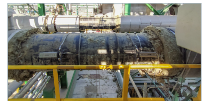
To set up the measuring point, the insulation only needs to be removed temporarily. The ultrasonic transducers are installed on the hot pipeline during ongoing operation.
