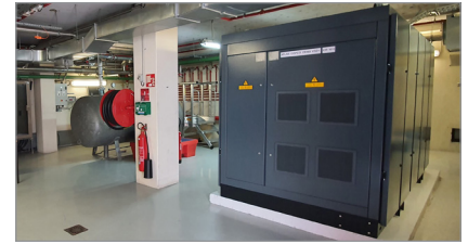
The compressor room
