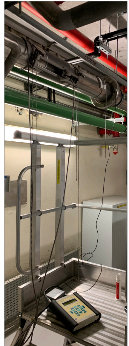
Temporary compressed air flow measurement with FLUXUS® G601
