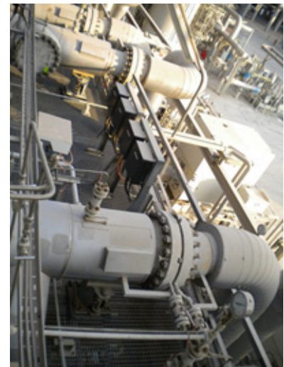
Rosemount Conditioning Orifice Plate installed
