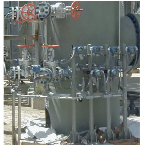
At-grade indication allows ease of access for technicians.
