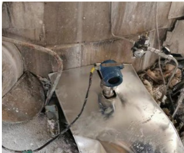
Rosemount 5408 Level Transmitter installed on a urea melting tank
