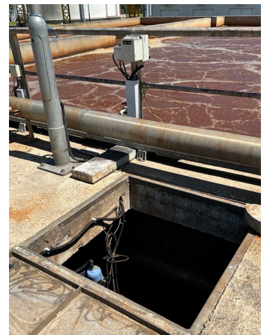
Image 1. The Rosemount™ 1208 Level and Flow Transmitter installed in a wastewater treatment basin
