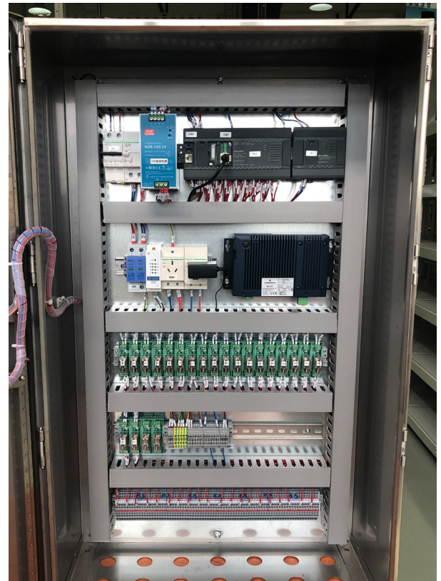
Dust Collector Control Cabinet
