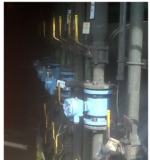
Installed Rosemount 8700 Magnetic Flow Meters at ArcelorMittal
