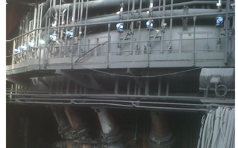
Installed Rosemount 8700 Magnetic Flow Meters to measure the cooling water flow at ArcelorMittal furnace
