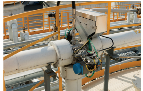
In-Line Distribution Valve installed on a piggable line enabling the transfer of finished product into a tank.
