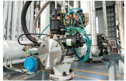
Head Line Distribution Piggable Valve installed at the end of a discharge header of a blender enabling pigging between the blender to storage.
